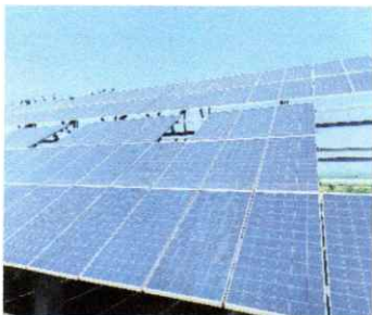
Solar PV installation on building roofs
