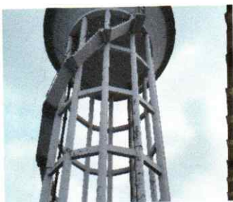
Water storage tanks
